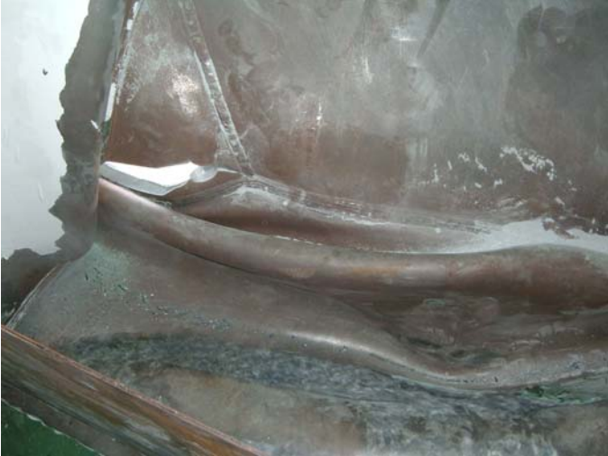
Fig 3: Internal damage in fwd store
