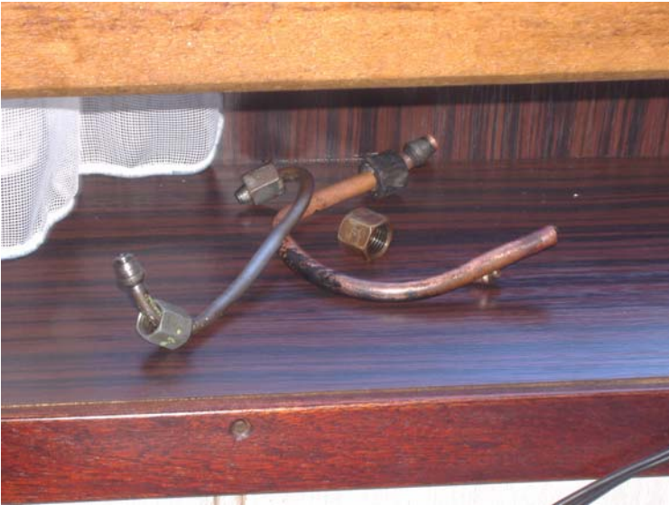
Figure 2: The copper instrument line which failed and an original steel instrument line removed from a similar gauge on Generator No 1.
