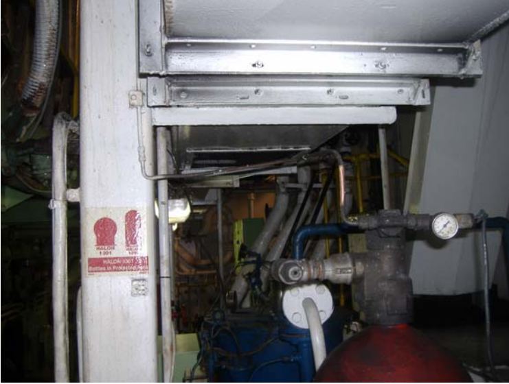
Figure 5: Copper pilot lines on Halon 1301 bottles.
