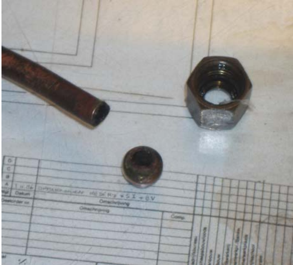
Figure 3: Close up of the failure site. Note the brazing of the compression fitting to the instrument line.
