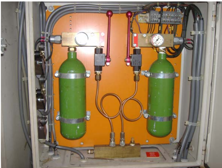
Figure 4: CO 2 Pilot Cylinders (discharged) for release of Halon into the Engine Room.
